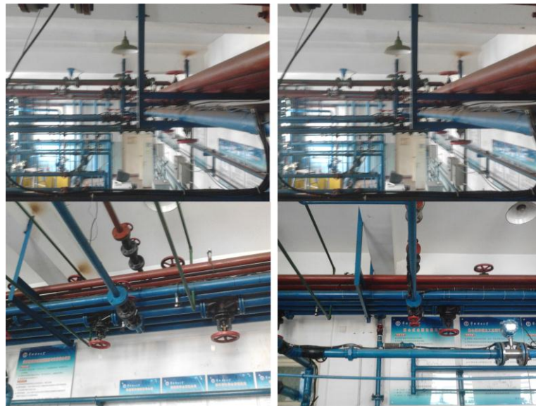
FIGURE 5 The photograph of pipe network
