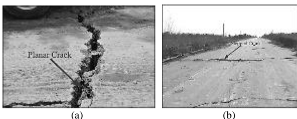
FIGURE 2 Shape of cracks. (a) Shape of planar crack; (b) Shape of stepped crack
